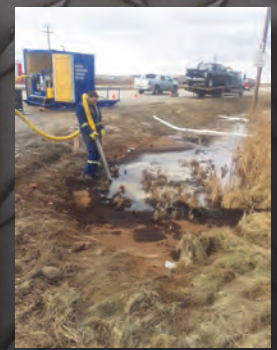
Diesel spill vac cleanup
