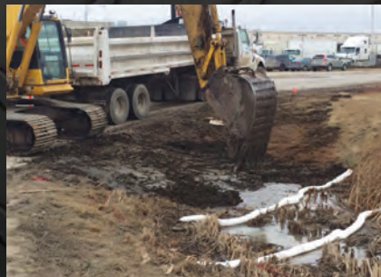
Diesel spill remediation
